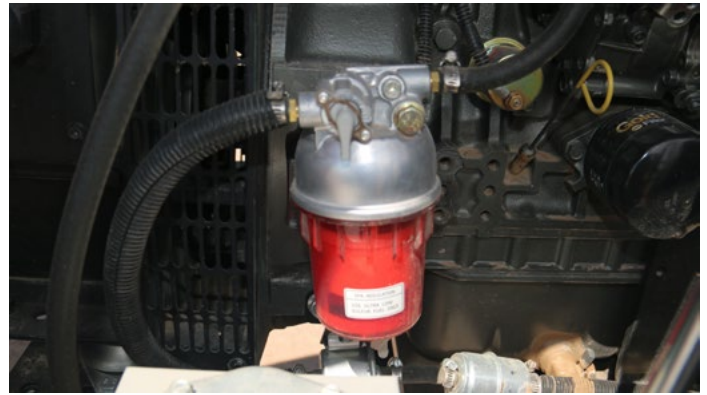
Check water separator
